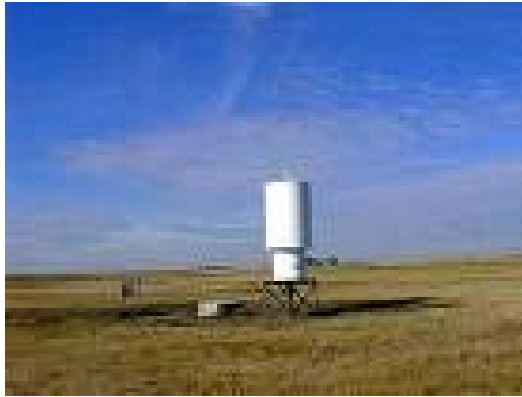
TACAN Beacon Antenna Figure 9
